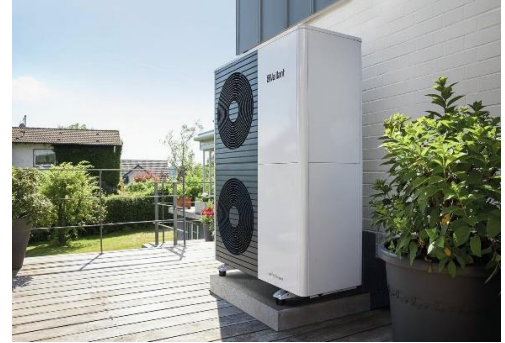
Typical Outdoor Residential Heat Pump Systems Equipment
